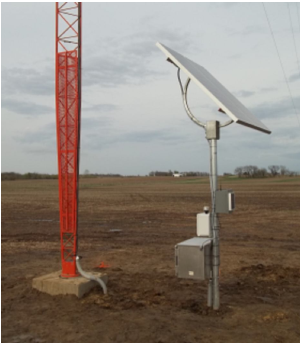
Power Generator with Custom Mount
